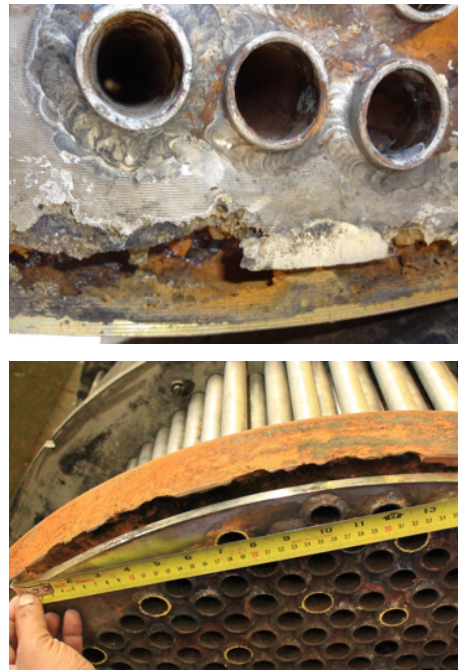
Figure 1: Crevice Corrosion on Tube Sheet Gasket Surface
