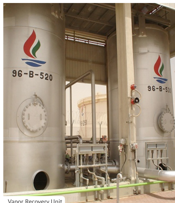
Vapor Recovery Unit
