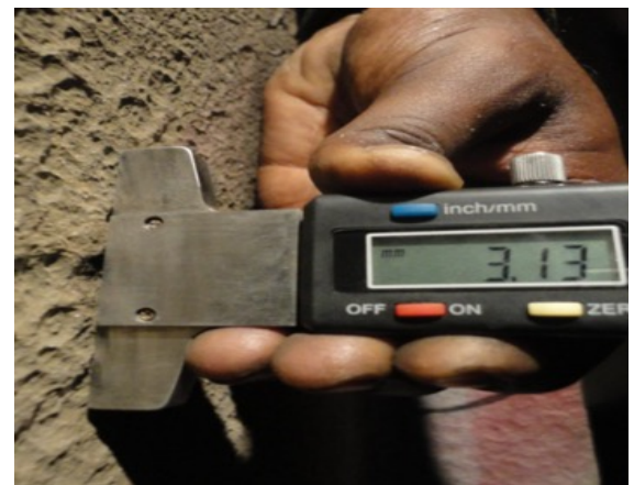
Figure 6. Acid gas enrich absorber Vessel shell deep pitting
