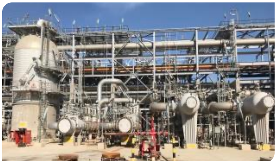
Feed Gas Filters & Dry Gas Filters
