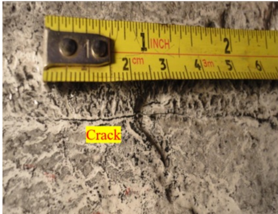
Figure 3b. Crack in the corroded area after Hydrogen bake out and prior to drum repair
