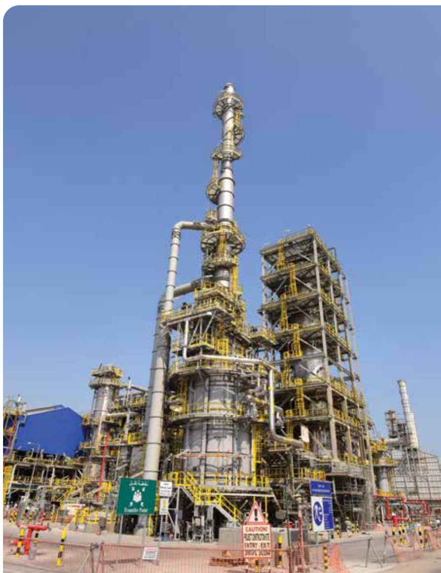
Gas Oil Desulphurization Unit (U-144) - MAA
