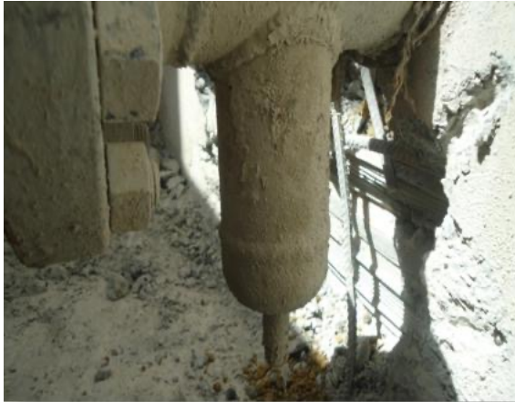
Figure 11. Drain boot in the pit. Internal corrosion (over 50% metal loss) in boot
