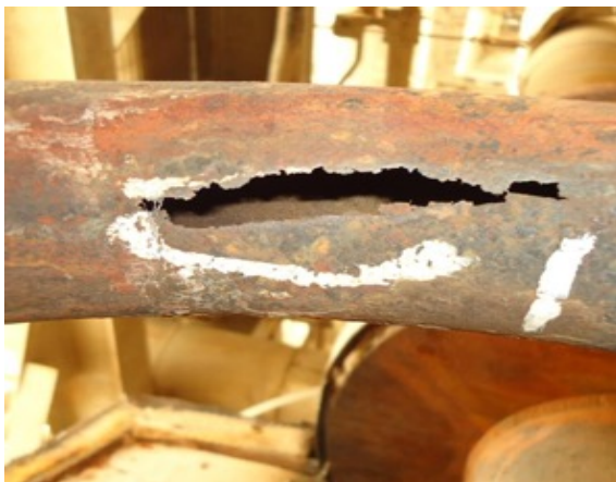
Figure 10. Waste heat boiler tube failure by external acidic gases in Incinerator section
