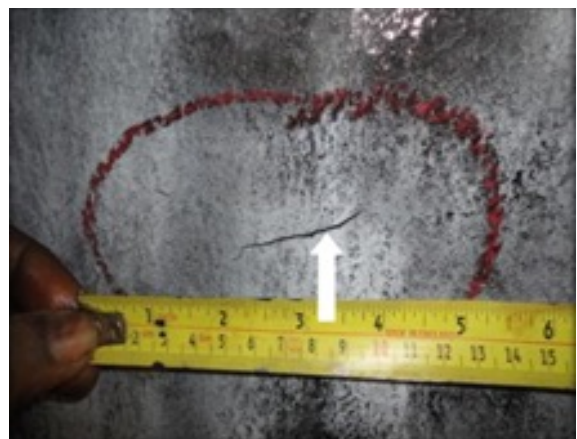
Figure 7. Cracks in shell material (CS) of a Lean/Rick Amine Exchanger
