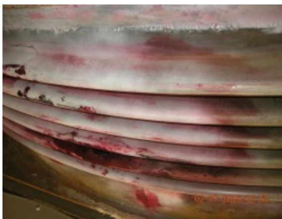
Figure 15. Perforations on expansion bellow (UNS S31603) connected to incinerator.
