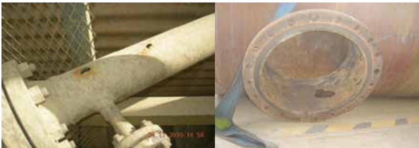
Figure 9. Internal corrosion of piping
