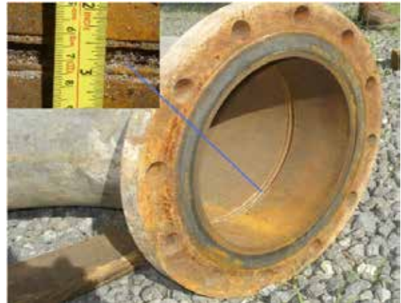
Figure 5. Flash corrosion in the CS piping downstream of the rich amine exchanger to stripper
