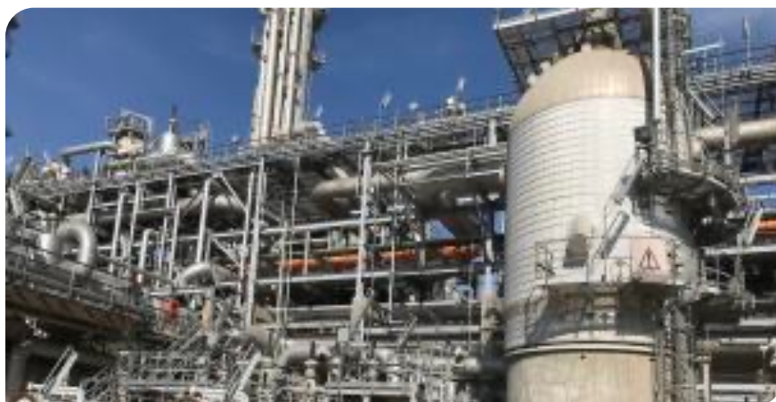
Mercury Guard Bed & After Mercury Filter
