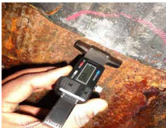
Figure 4. DEA Stripper tower interface between SS clad and CS. 4~5 mm metal loss at the interface due to galvanic effect and erosion - corrosion
