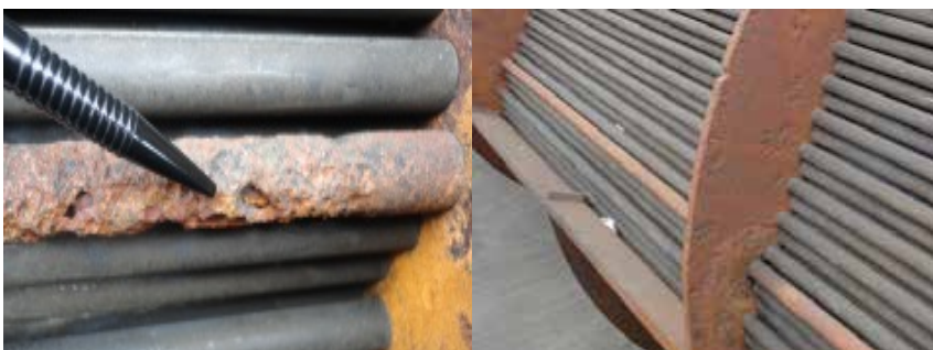
Figure 14 a & b. Perforation of tie-rod and sleeves (galvanic corrosion). Localized corrosion and enlargement of baffle plate holes
