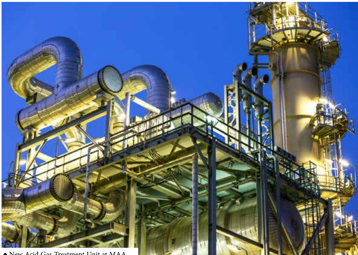
• New Acid Gas Treatment Unit at MAA
