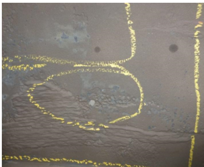
Localized corrosion characterized by pitting, grooving and erosion
