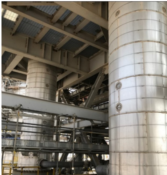
(Vertical exchanger: Crude Overhead / Crude)
