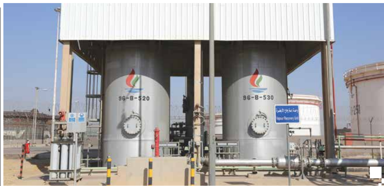
Vapor Recovery Unit at Al-Ahmadi tank-farm
