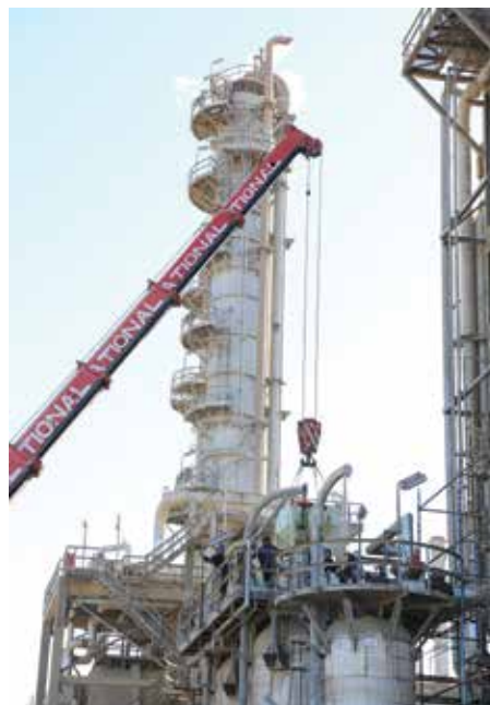
MAA Refinery Departments demonstrated an outstanding performance during the FY
