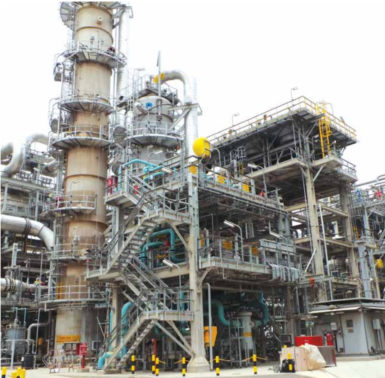
Acid Gas Exhaust Unit
