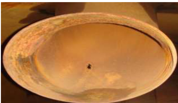
Severe Corrosion / Thinning & Perforation in 90 Internal Elbow on Inlet Nozzle "N1"
