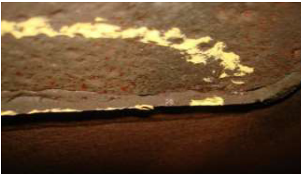
Corroded impingement plate fillet weld
