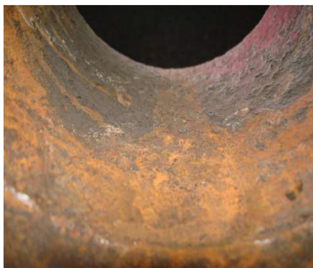
Internal corrosion of liquid inlet nozzle
