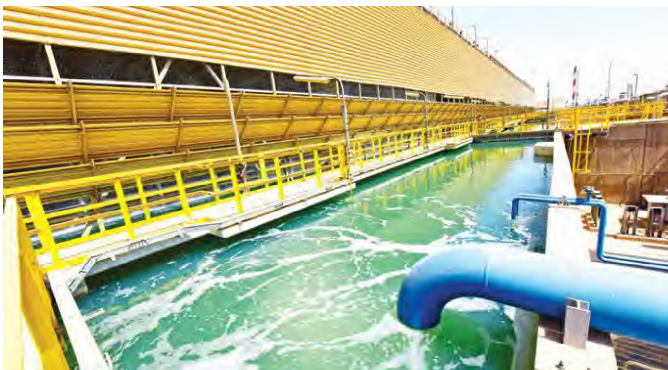
Effluent sea water is another source of H/C loss
