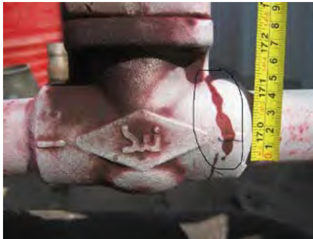
Fig. 7: Recycle hydrogen line cracks.
