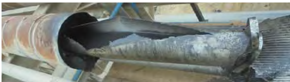
Fig. 1a: The rupture pipe as found condition on the pipe rack
